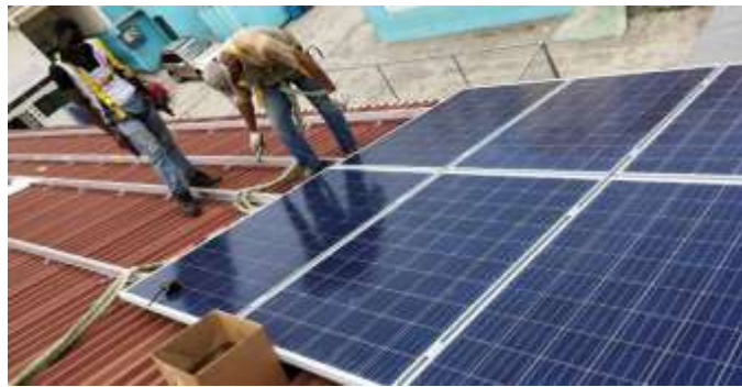
Figure 2: Solar panels being installed on the roof in St Andrew Settlement, Jamaica (UNDP, 2017)
